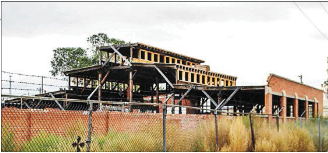
A variety of tenants have already shown interest in taking up space in the mixed-use location.
